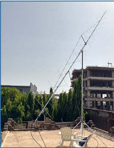
The flat roof of a service building was a suitable spot to install the EME antenna.
