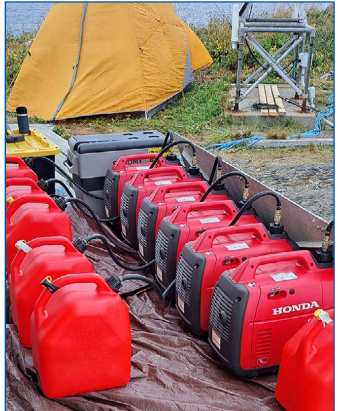
"St. Paul Power & Light" generators.
